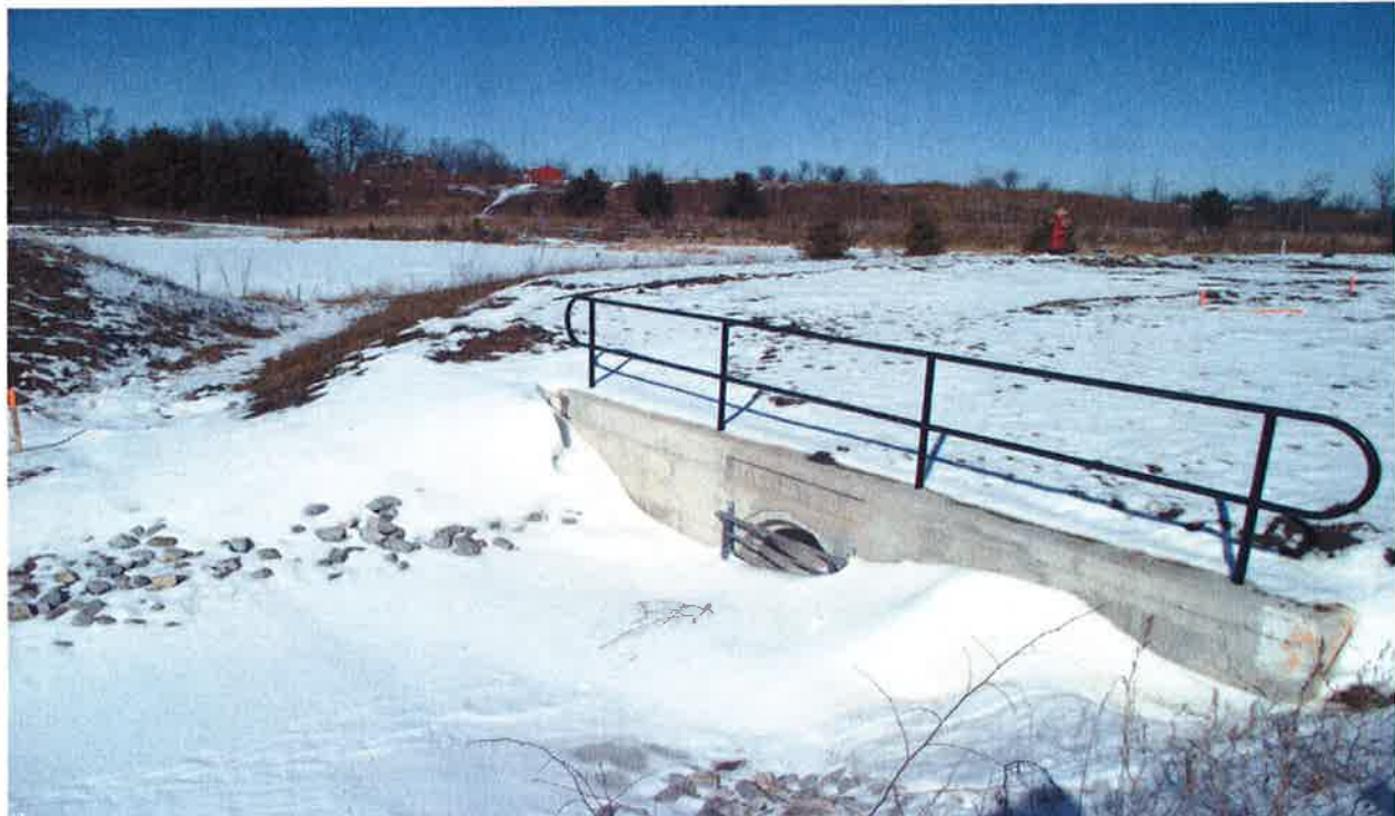
Mayfield Road\Section4: Concrete culvert and Storm Water Management Pond at the Northeast Corner of Mayfield Rd. and Kennedy Rd. Intersection.
