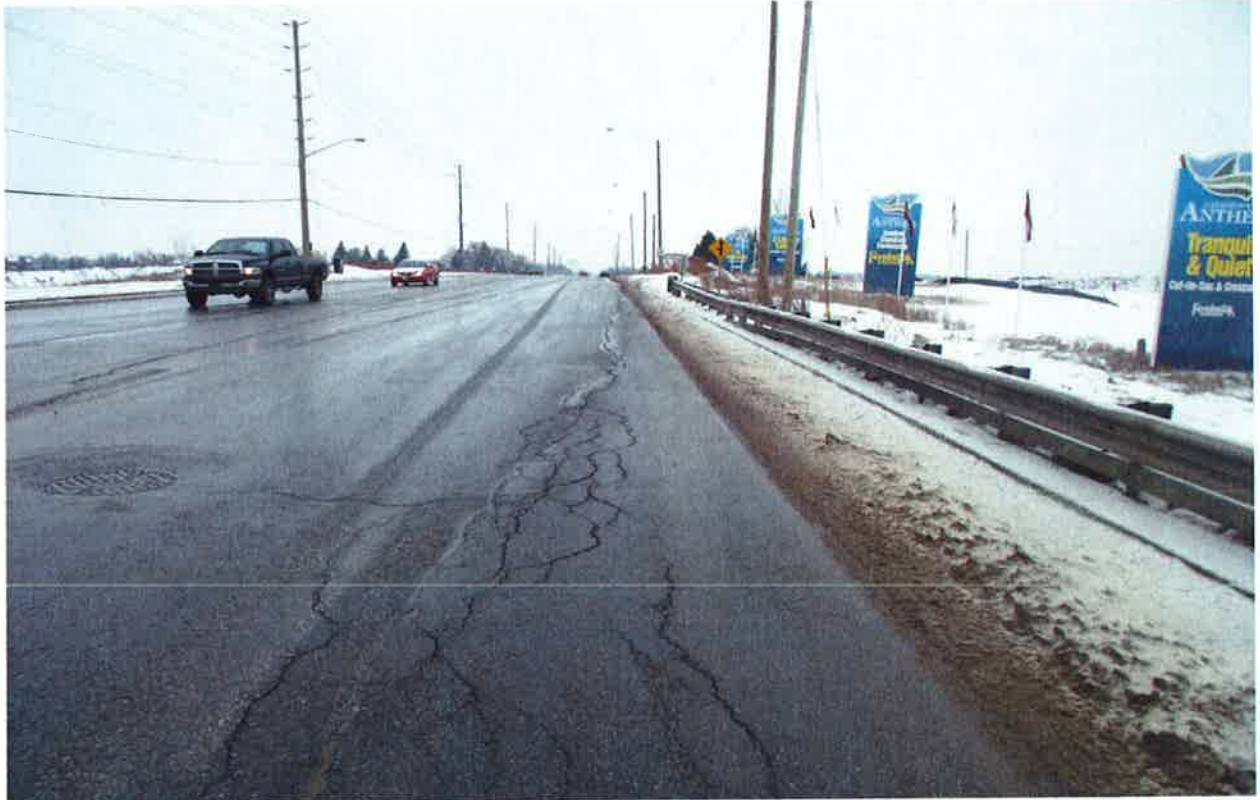
Mayfield Road\Section4: Looking towards West \ from Kennedy Road to 150 m Westerly\see cracks and distortion area\ new Subdivision will be constructed at the Northside of Mayfield Rd., West of Kennedy Rd.
