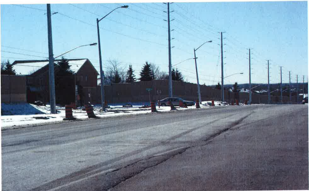
Mayfield Road\Section4: Looking towards West\cracks and Distortion Area \See Noise Wall along the South Side of Mayfield Road
