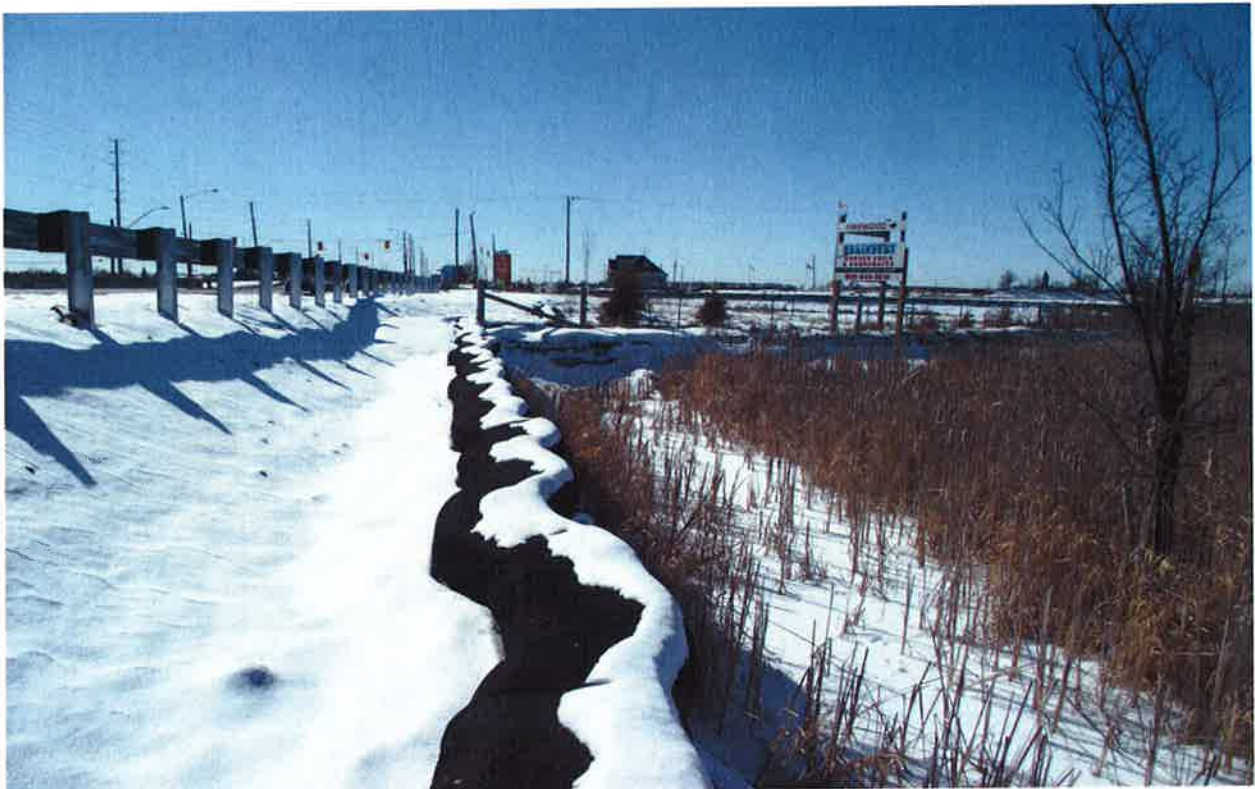
Mayfield Road\Section4: Looking towards West\Steel Sheet Piles at the North Side of Mayfield Rd and Wetland Area to the North OF Mayfield Rd and East of Kennedy Rd.
