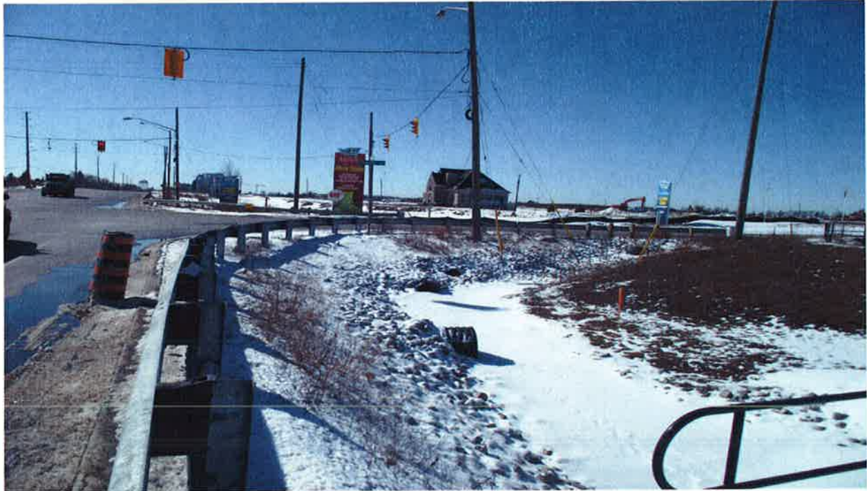
Mayfield Road\Section4: Looking towards West\ Culverts and wetland at the Northeast Corner of Mayfield and Kennedy Rd. Intersection.
