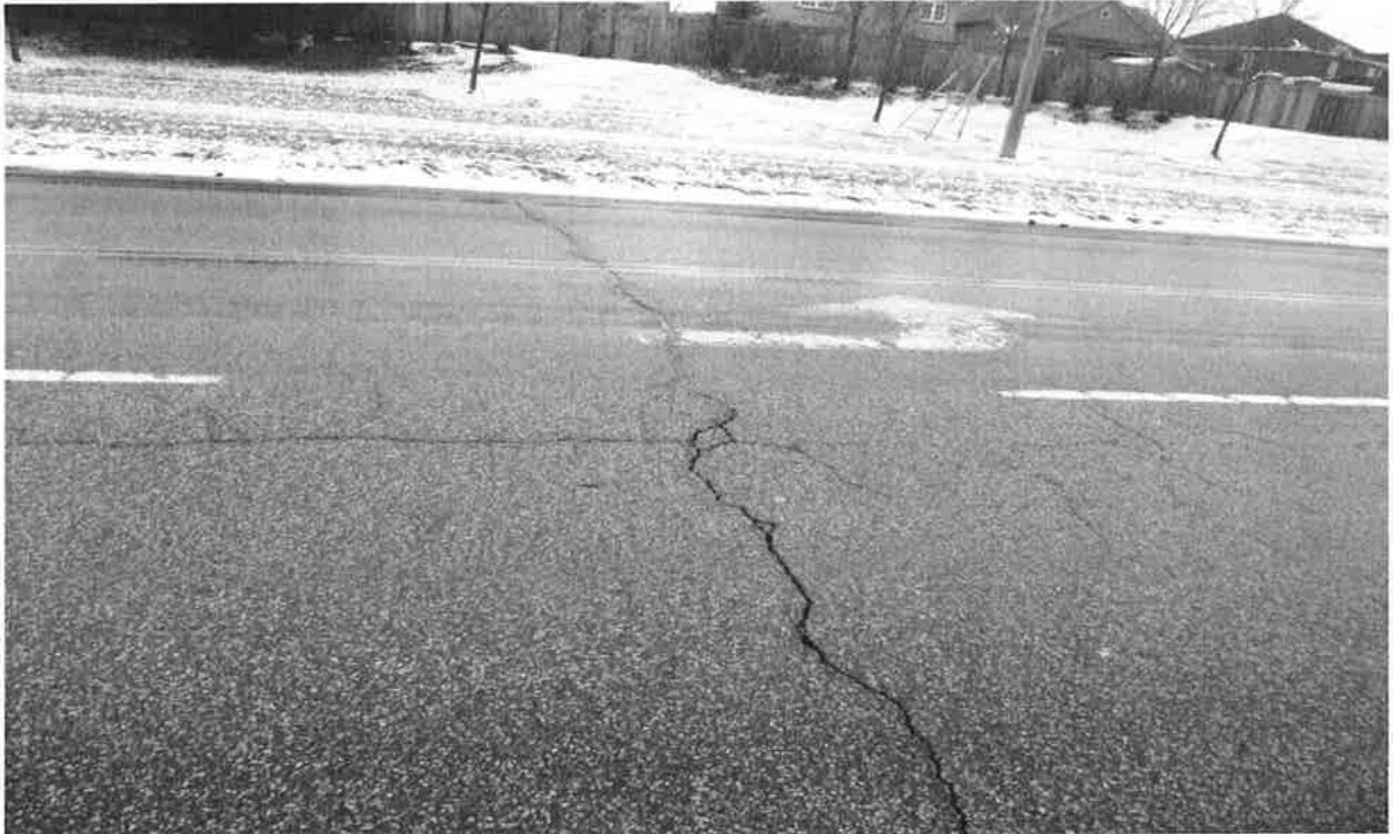
Mayfield Road\Section 2: Cracks on the Pavement
