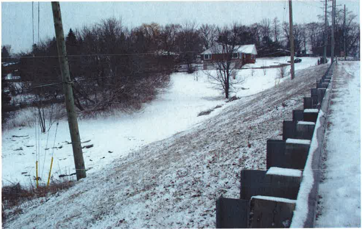
Mayfield Road\ Section 3: Looking towards West\Embankment Fill west of the Structural Bridge \ South side of Mayfield, West of the Bridge
