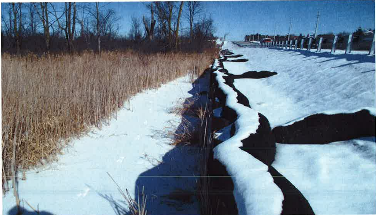
Mayfield Road\Section4: Looking towards East\Steel Sheet Piles at the North Side of Mayfield Rd. as Retaining walls for the road Embankment (Approx. 400 m long)
