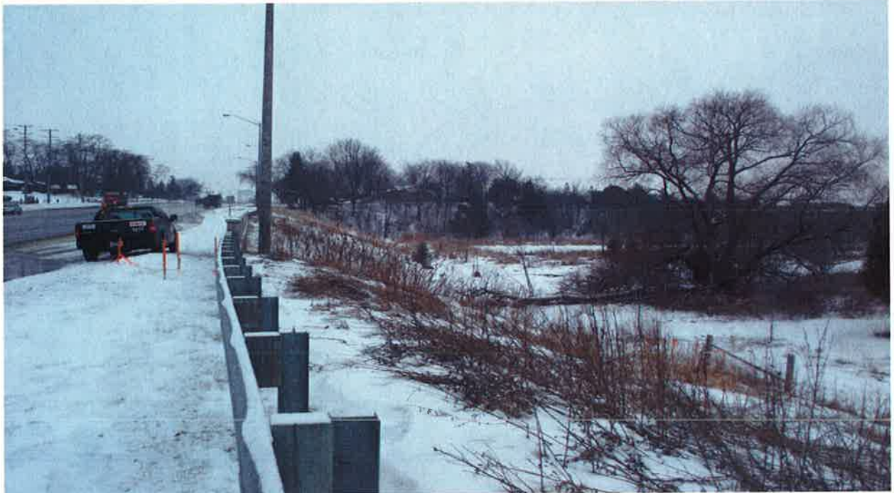
Mayfield Road\Section 3: 700 m West of Kennedy Road Looking towards West\Embankment Fill for Structural Bridge crossing Tributary
