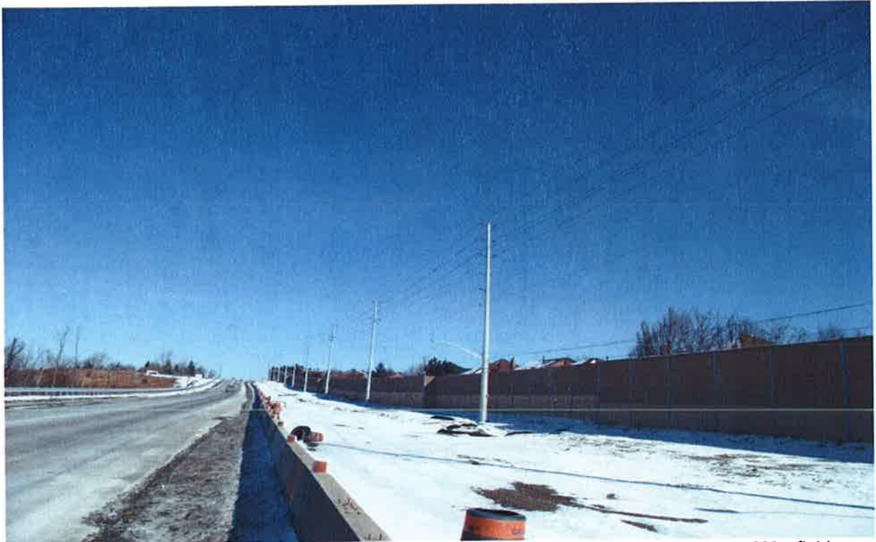
Mayfield Road\Section4: Looking Towards East\Widening Construction for the Southside of Mayfield, East of Kennedy Rd.
