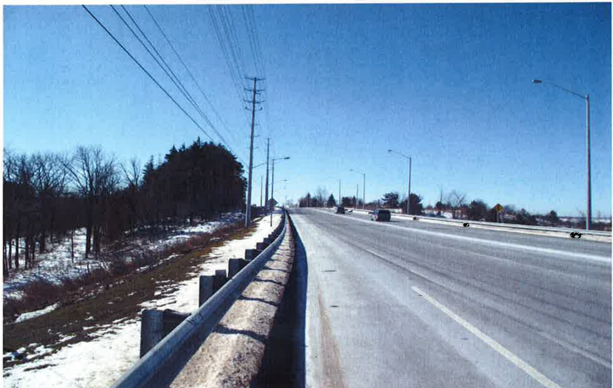
Mayfield Road\Section 5: Looking towards West\South side of Mayfield Rd., High Fill Embankment
