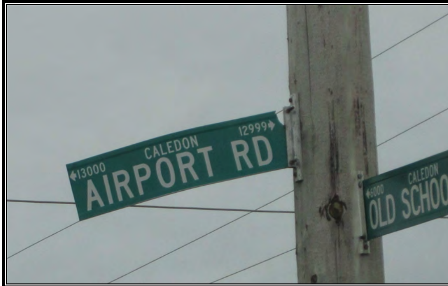
Figure 7: Damaged Street Name Sign Airport Road at Old School Road
