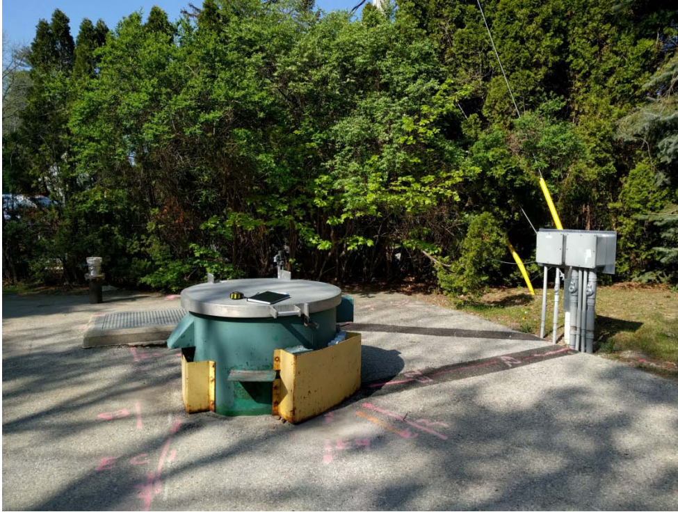
Plate 5: View of the Indian Road SPS, wet well and pump, looking southwest.
