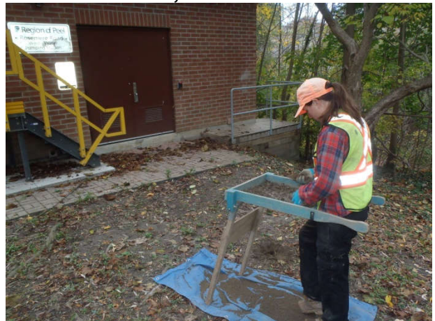
Plate 4: View northeast, showing crew test pitting adjacent to structure at Rosemere Road SPS study area.
