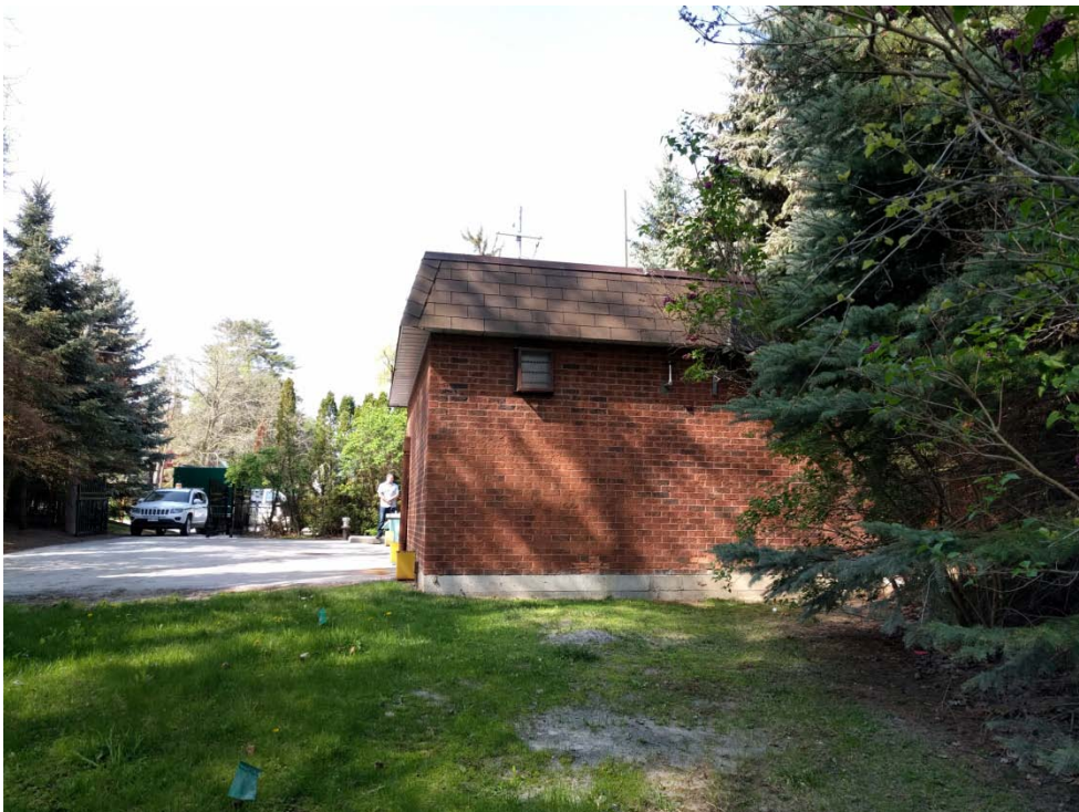
Plate 4: View of the Indian Road SPS diesel generation and control building, from rear of property, looking south.
