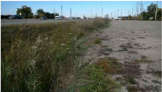
Photo 3. Roadside ditches with no direct connection to watercourses or fish habitat at northern extent of project area (Oct 22, 2018).
