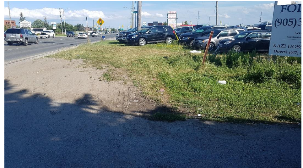
Image 6: View of disturbances associated with the asphalt roadway and driveway, concrete curb, paved shoulder, previous grading activities and buried utilities.
