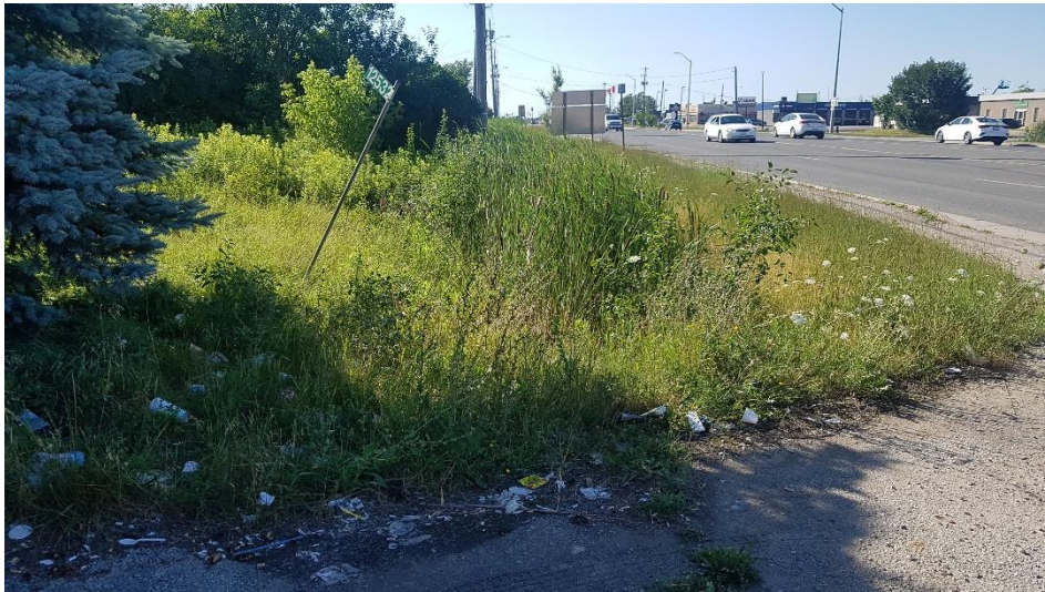
Image 5: View of disturbances associated with the asphalt roadway and driveway, paved shoulder, culvert and wet ditching.
