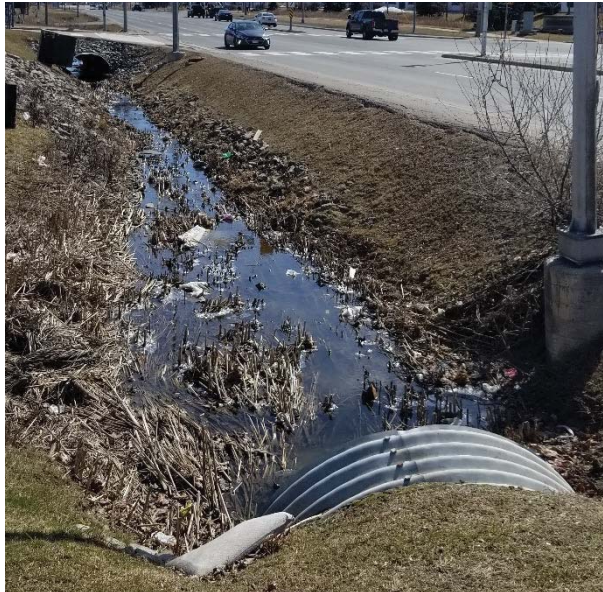
Photo 31: A corrugated steel culvert was observed at the entrance to 12275 Highway 50, where an RV sales and servicing center was located. The drainage ditch shown flows to the south on the east side of Highway 50.
