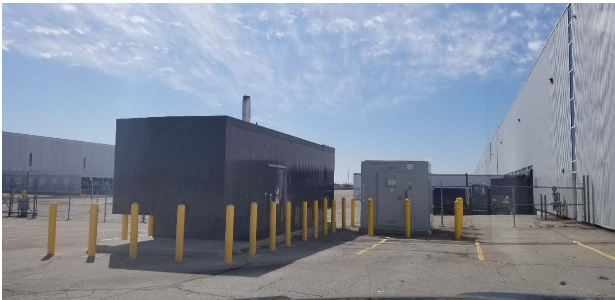
Photo 30: A large commercial warehouse and trucking terminal was observed at 86 Pillsworth Road. At the south of the building in the central region a large pad transformer and possible generator were observed.
