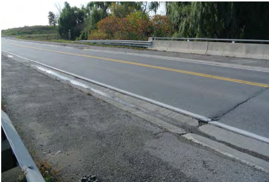
Plate 6: View of the bridge deck, concrete drainage system, asphalt shoulders, and concrete railing system, looking southwest.
