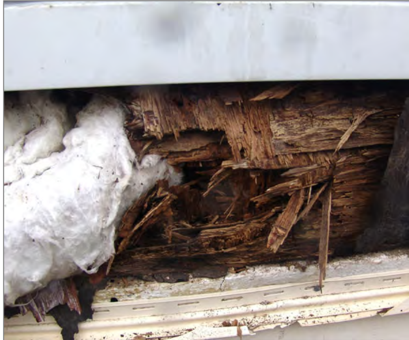
Above: Delaminated plywood and insulation under the exterior siding, 2011
