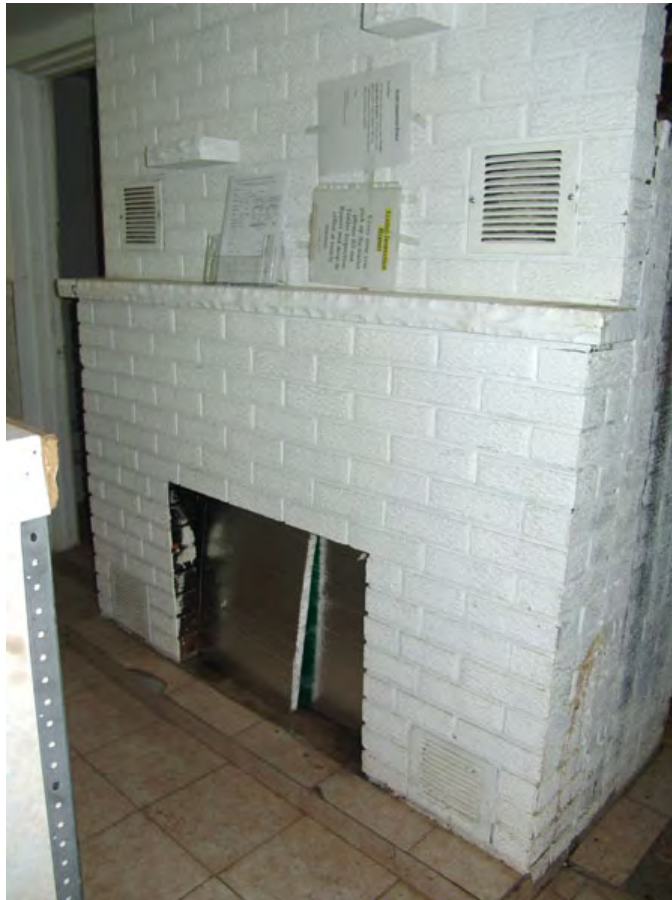
Above: Interior of ground floor looking northwest from entrance on south facade.
