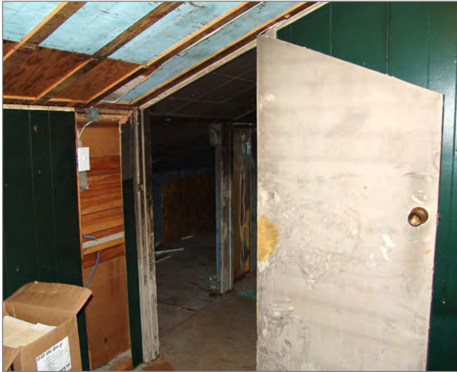
Above: Second floor, north room, looking southeast toward stair landing (C) and inside crawl space (L)
