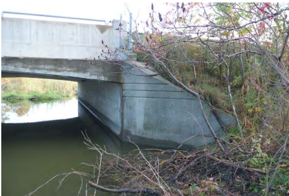
Plate 10: Detail of south abutment, looking east. Note the horizontal fluting on the wingwall.
