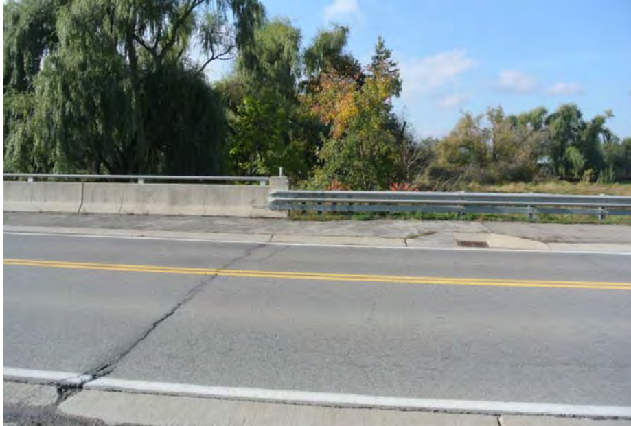
Plate 7: View towards the railing system and metal barrier system located on the west side of the bridge, looking west.
