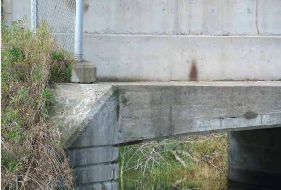
Plate 11: Detail of the abutment, deck, and concrete railing system on the southeast side of the bridge.
