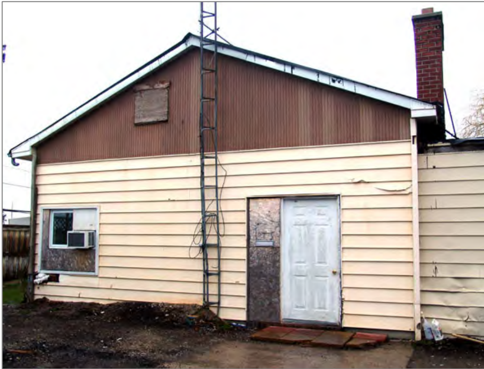
Above: South facade. The massing (width) of the main structure is broad, suggesting the roof has been raised and/or extended east, 2011.
