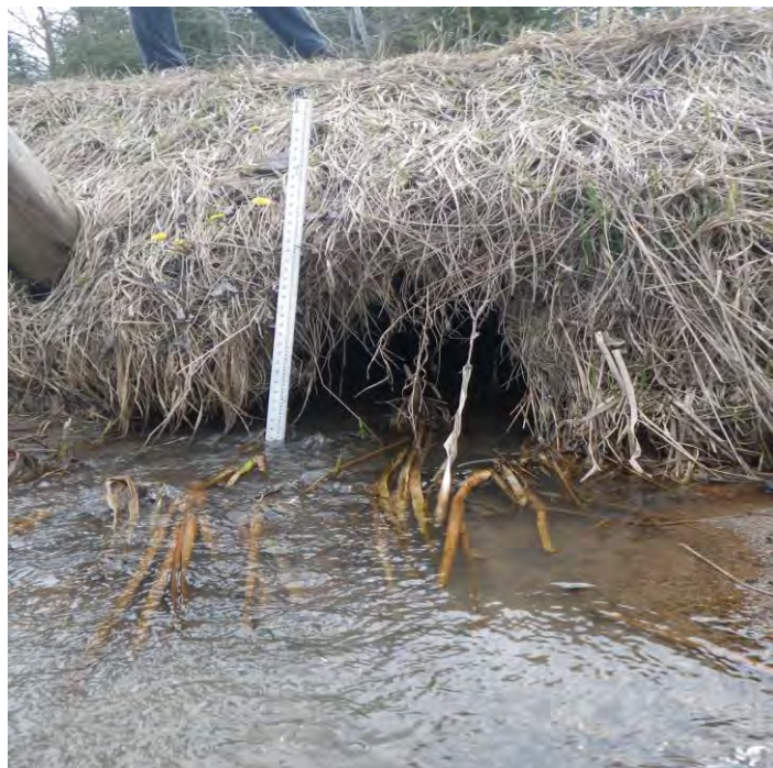
Photo 16: View looking upstream towards culvert outlet which is being compromised due to slumping bank.
