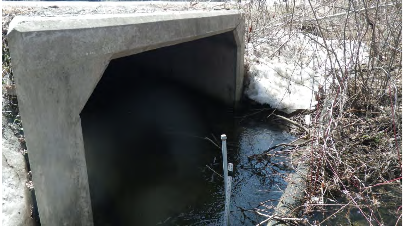
Photo 19: View looking downstream at culvert inlet. Level logger is present just upstream of culvert.
