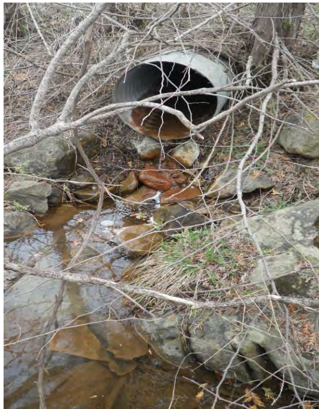
Photo 14: View looking upstream towards the perched culvert outlet.
