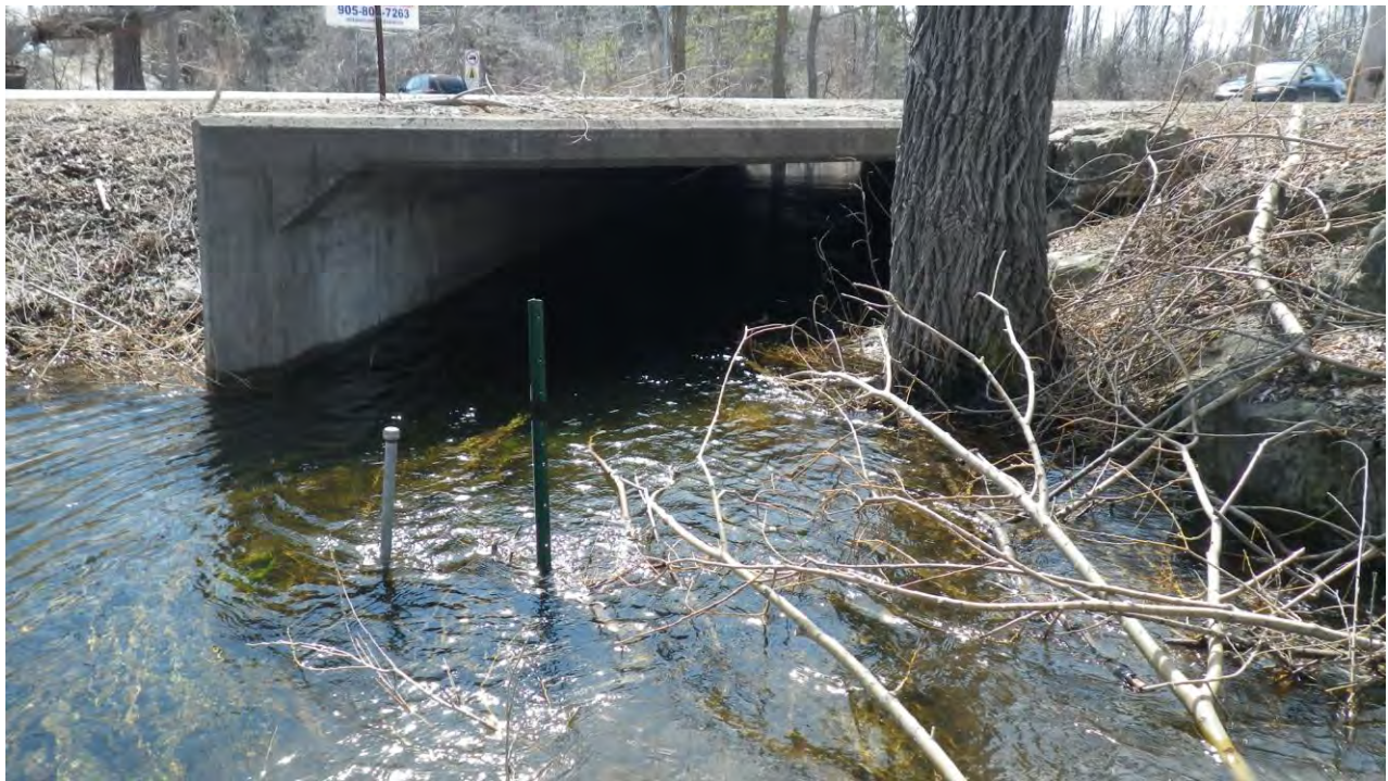
Photo 21: View looking downstream towards culvert inlet. Level logger is present just upstream of culvert.
