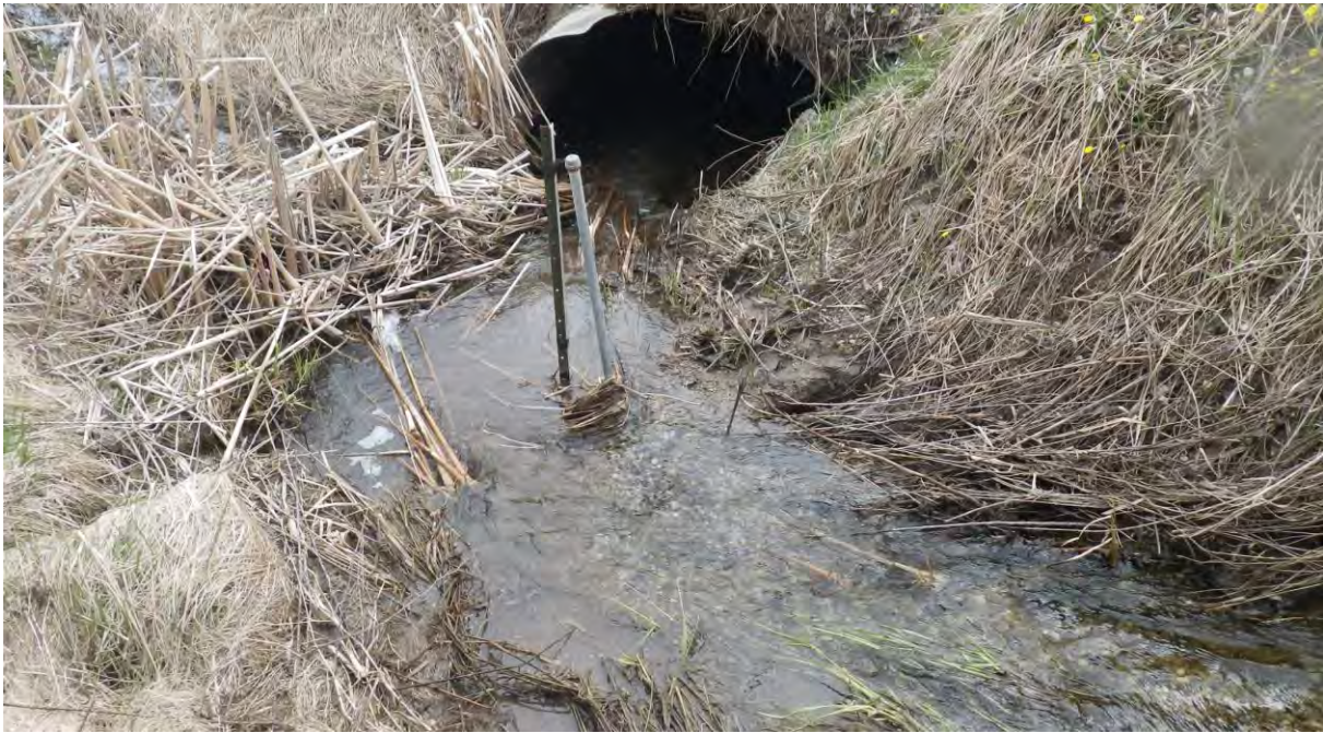
Photo 11: View looking downstream towards culvert inlet. Level logger is present just upstream of culvert.
