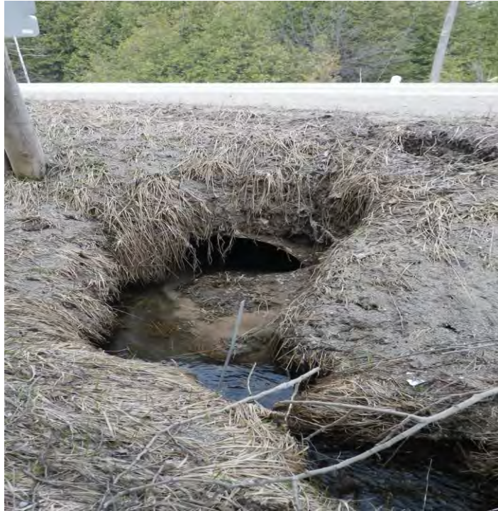
Photo 15: View looking upstream towards culvert inlet which is being compromised by the failing bank.
