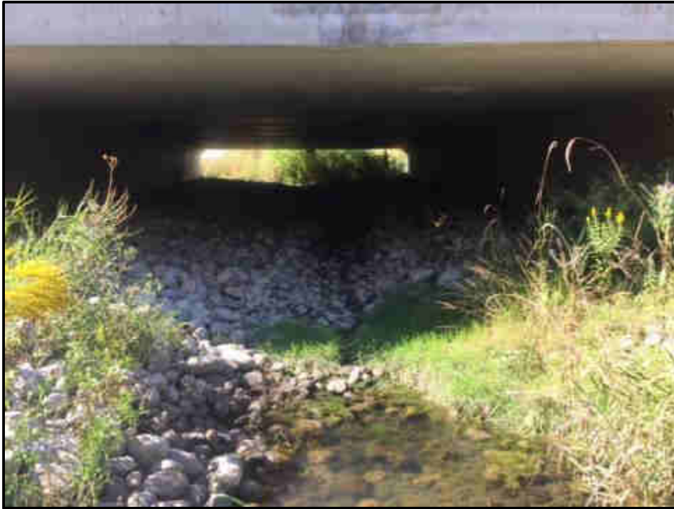
Photo 1. Mullet Creek – Looking West through the Culvert from Downstream * Instream Culvert Dry
