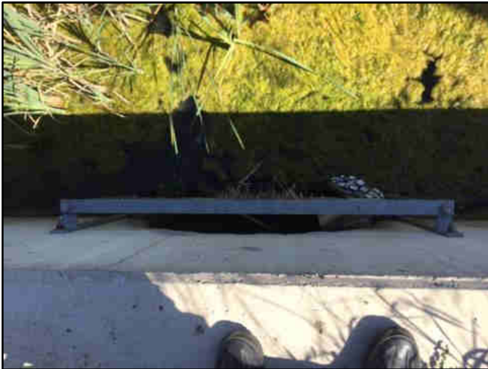
Photo 16. Drainage Feature #6 – Standing Water at Culvert Outlet
