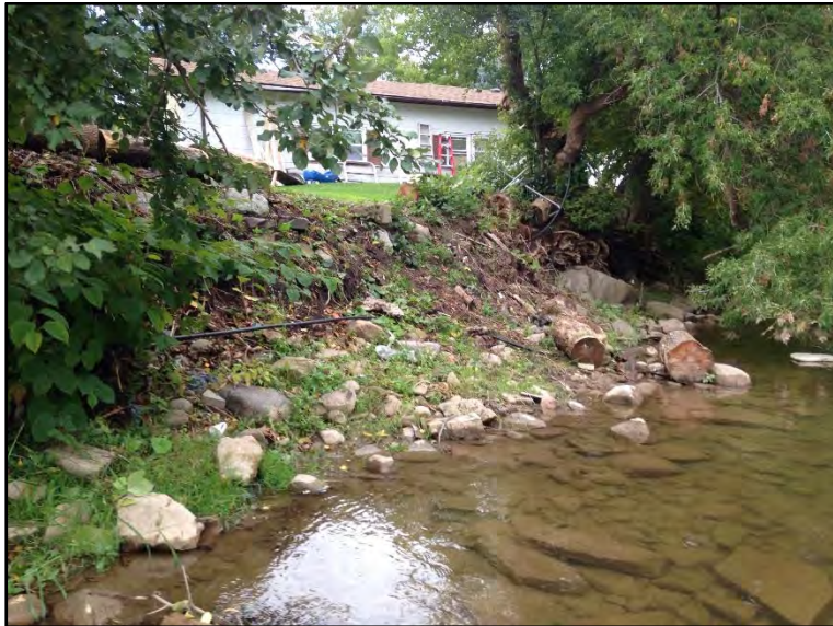
Photo 19: 0-200 m downstream reach, pollution and bank erosion on right bank.
