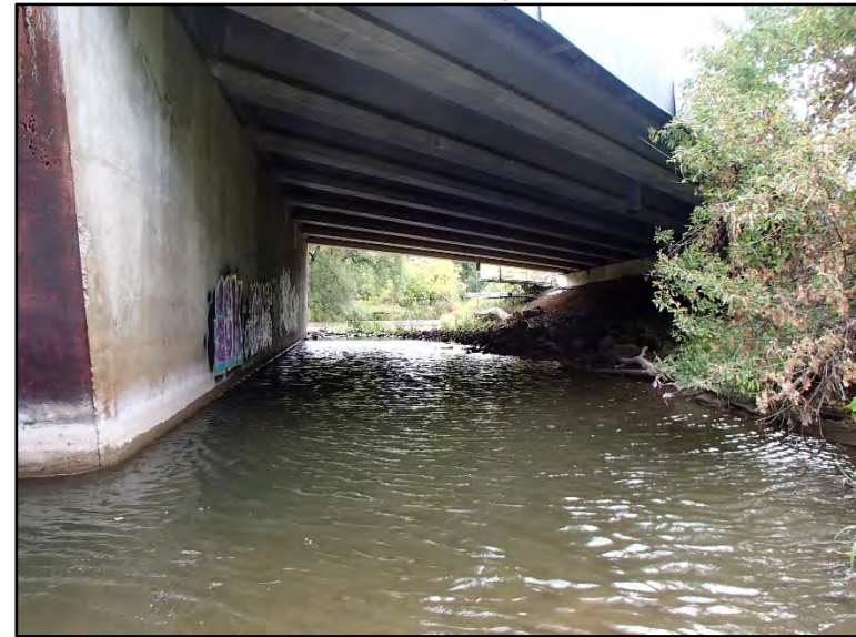
Photo 8: ROW channel on south side of southern pier (right channel). Photo looking downstream.
