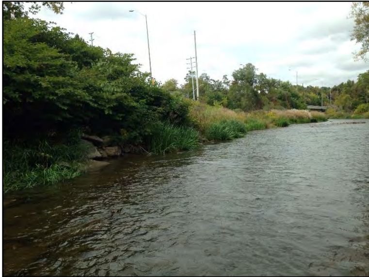
Photo 17: 0-200 m downstream reach, right bank immediately upstream of gabion wall and river-front residential properties.
