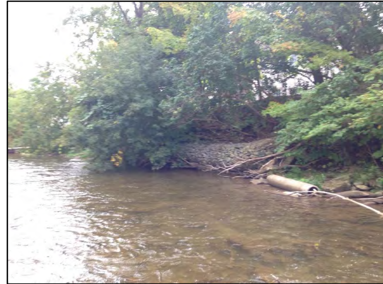
Photo 18: 0-200 m downstream reach, gabion wall erosion protection.
