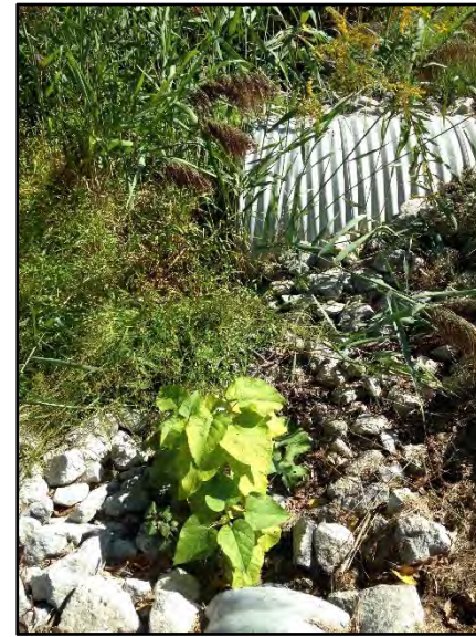
Photo 8: Looking down at outlet of CSP parallel to Mississauga Road passing under a driveway north of C2 on east side.
