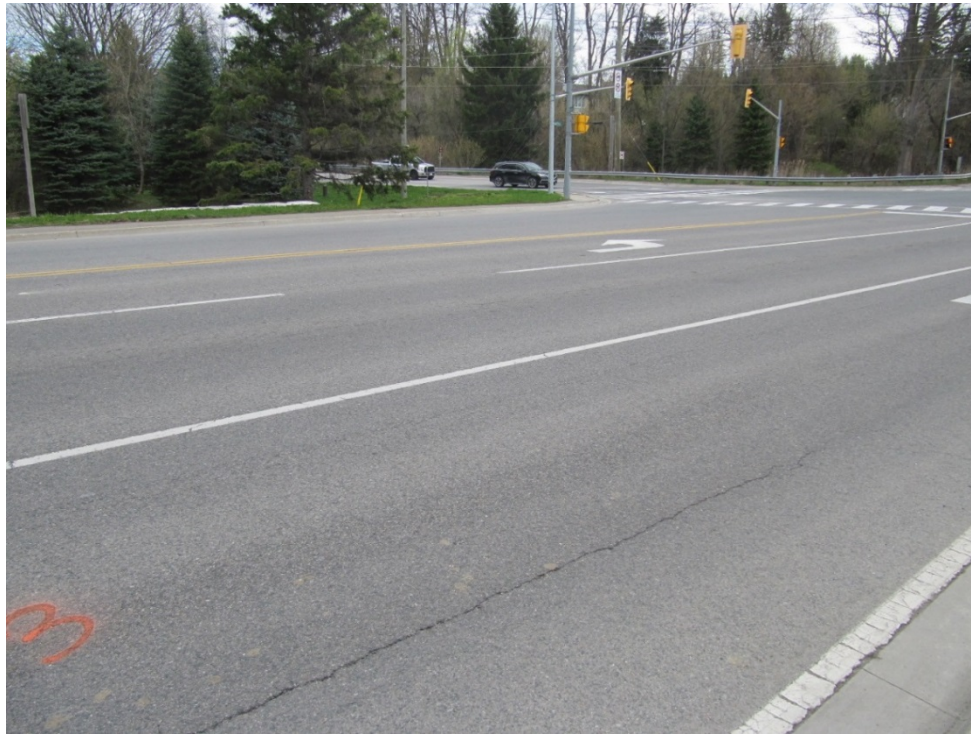
Photo 3: Longitudinal construction joint opening on West leg of intersection
