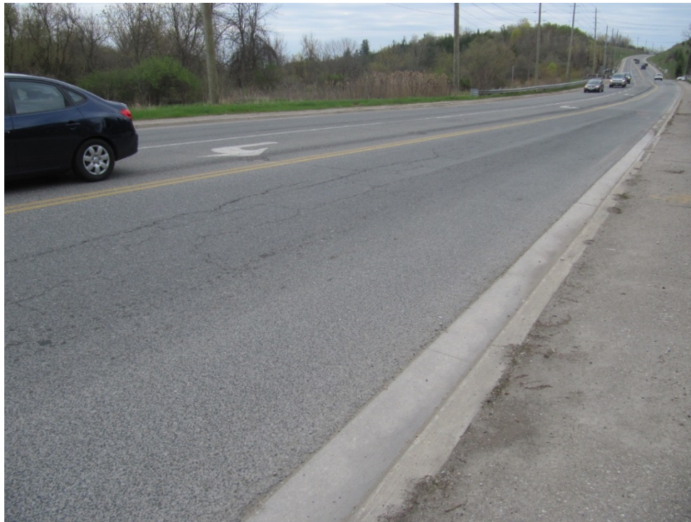
Photo 2: Alligator cracking on South leg of intersection
