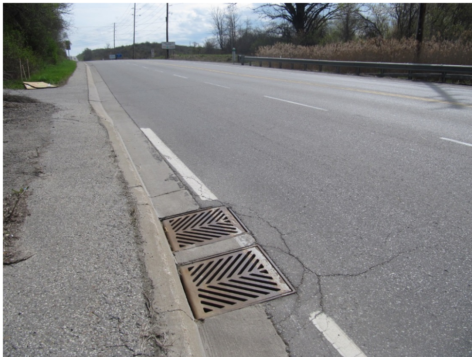
Photo 4: Pavement edge cracking on East leg of intersection
