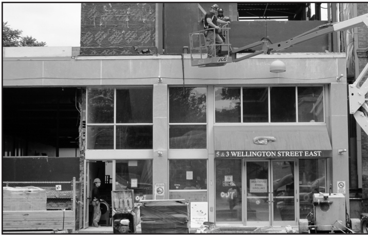
Workers look over blueprints for the new Members Lounge on the second floor of the new Art Gallery. Construction of the gallery's loading door (far left) is well on its way.
