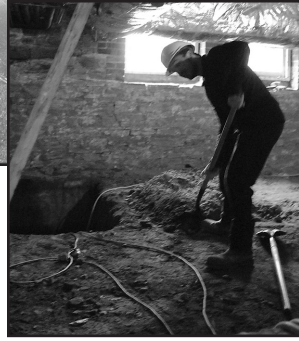
We are moving along nicely! This is the current state of the Courthouse basement—in our last issue of Strata we showed the same room at the start of our excavation (right).
