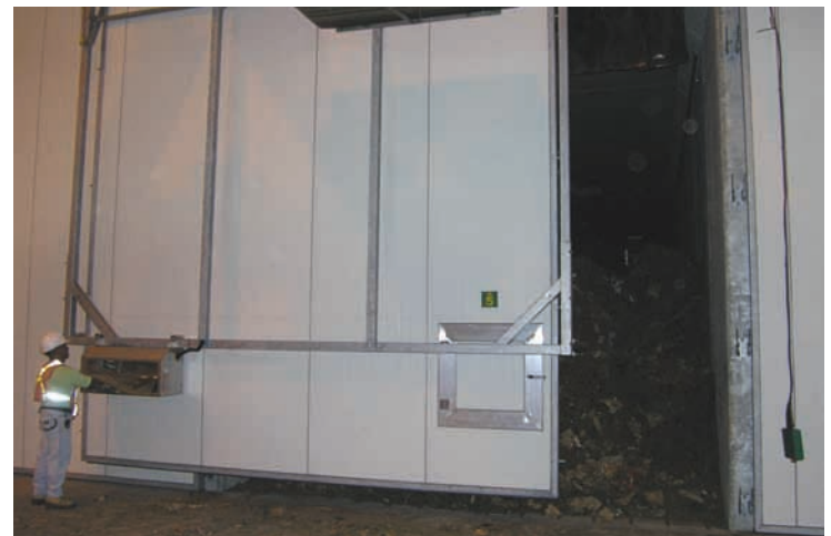
Composting cell at Peel IWMF Organics Plant
