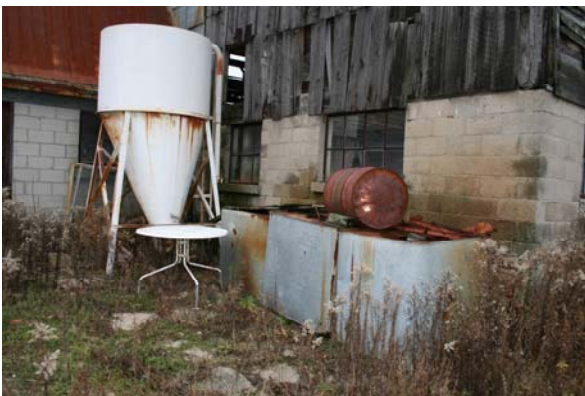
Photograph No. 5 Empty containers on east side of Building B.
