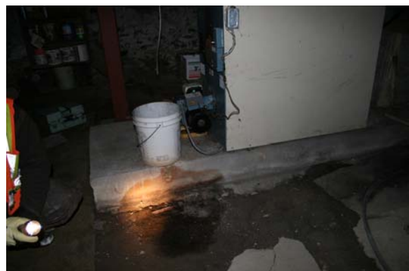
Photograph No. 12 Oil-fired furnace in basement of Building A.
