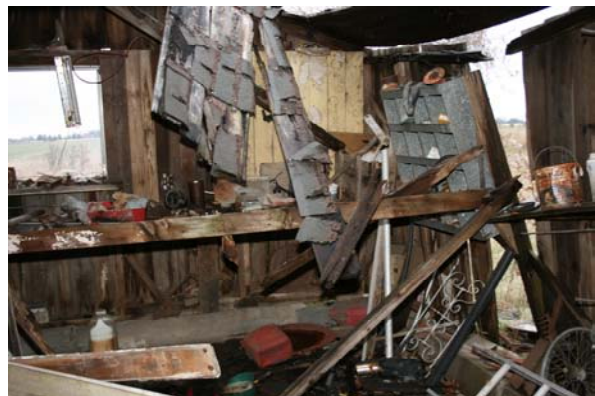
Photograph No. 6 View of damaged Building C. Building used for general storage.
