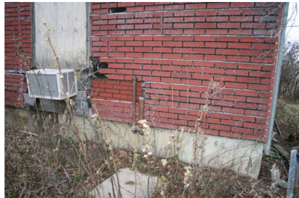
Photograph No. 10 Air-conditioning unit and fill and vent pipes on southeast side of Building A.
