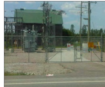
Hydro One Networks Station
