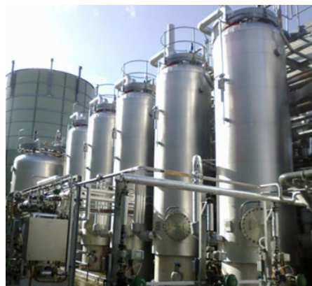
Figure 3-4 THP system at Davyhulme, UK
