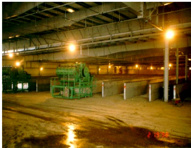
Figure 3-16 In-Vessel, Horizontal Agitated Bin, Composting Facility
