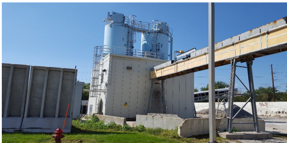
Figure 3-12 Lime Stabilization System
