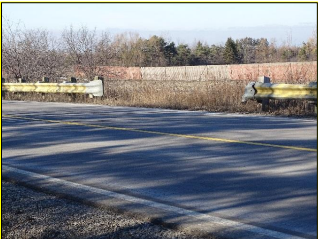
Figure 34: Steel Guide Rail Leaving-End along Countryside Drive
