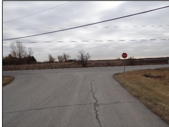
Figure 28: Missing Checkerboard Sign (Countryside Drive and St. Johns Road)
