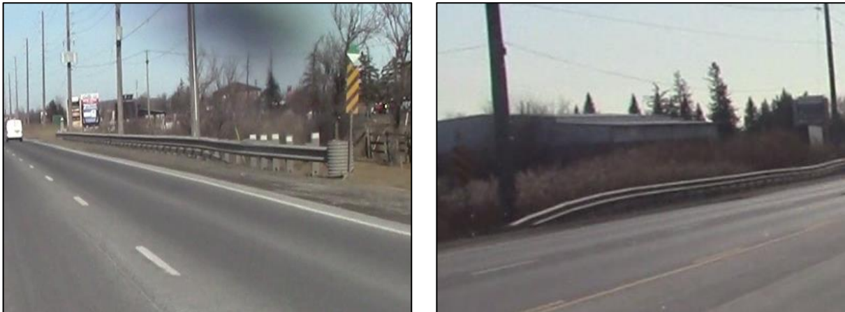
Figure 35: Missing Crash Cushion along Regional Road 50
