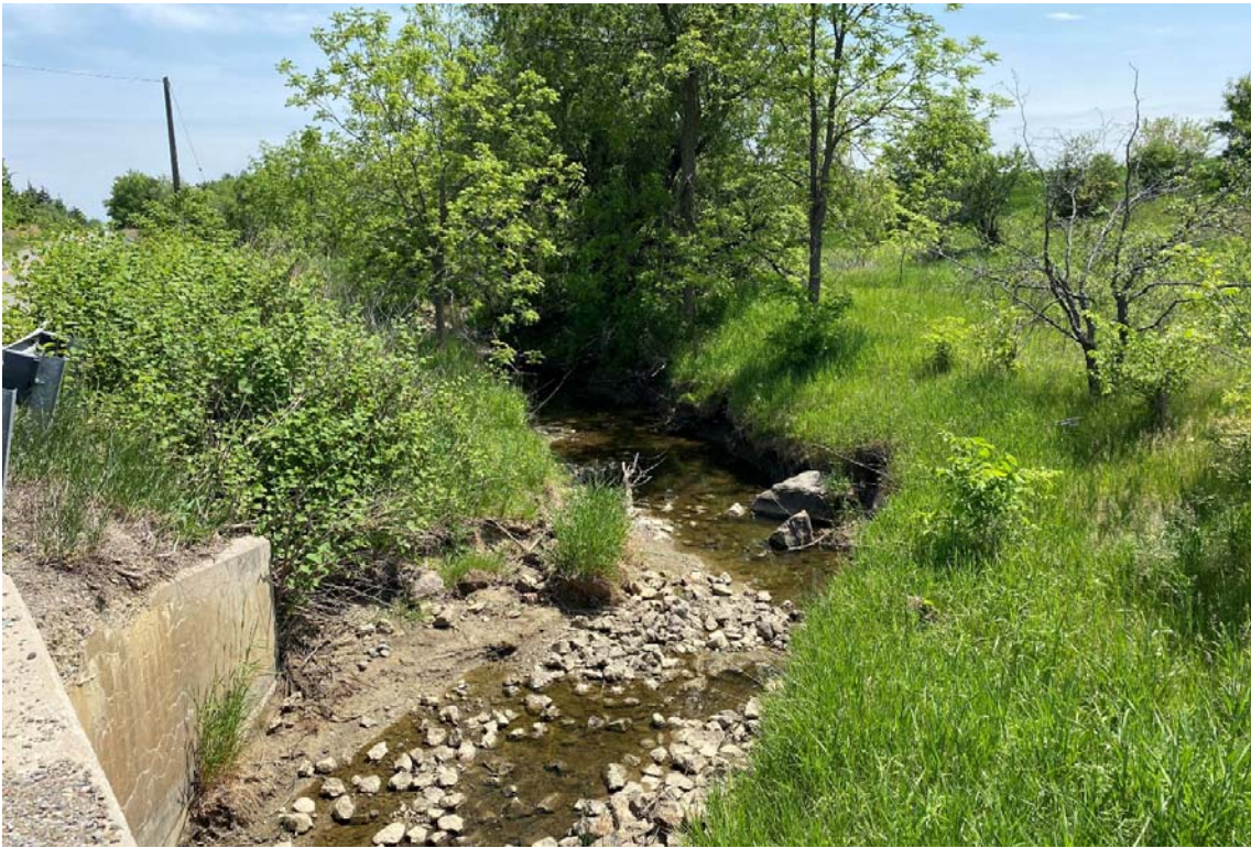
Image 8: Looking south. – Clarkway Tributary as it enters to the west side of Clarkway Drive. Riparian vegetation and cross section of creek are in much better condition with an increased localized capacity for both aquatic and terrestrial ecological function.
