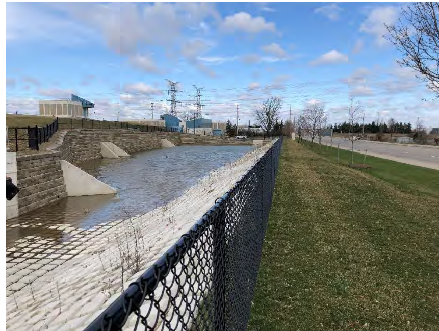
Plate 2: Northwest view of the pumping station and grassed lawn; Area is disturbed, no potential
