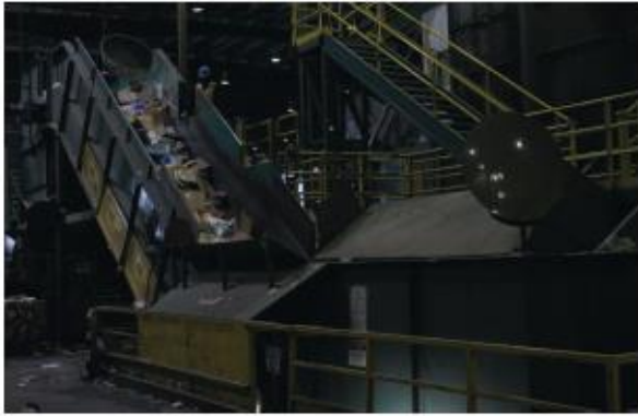
Before: Light fixtures with 400W bulbs
