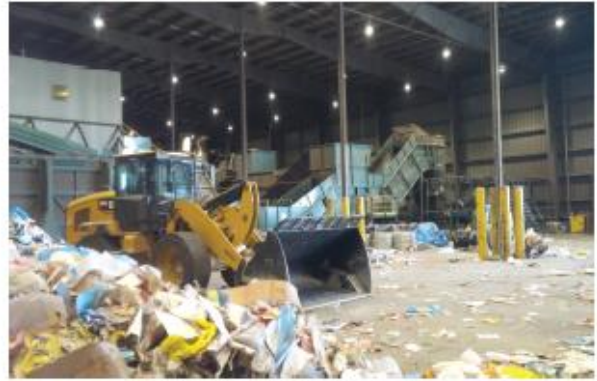
After: Combination of 200W and 100W integrated LED light fixtures. Illumination is 10 times brighter!
