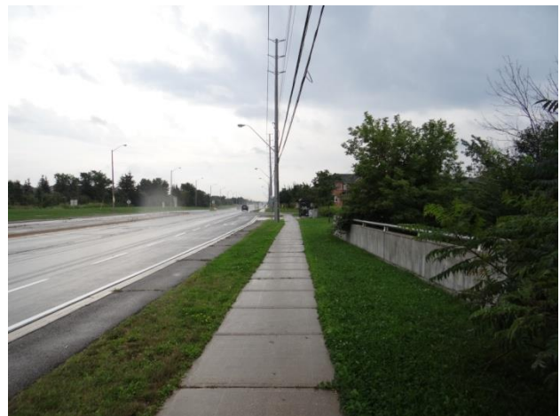
Plate 10: Sidewalk at center with culvert headwall at right on west side of Airport Rd., looking south.
