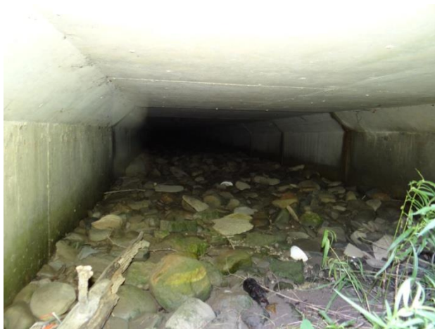
Plate 11: Concrete culvert carrying Humber River under Airport Rd. south of Yellow Avens Blvd, looking east.
