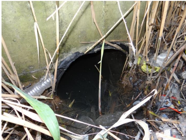
Plate 7: East headwall of pipe culvert carrying Humber River under Airport Rd., looking west.
