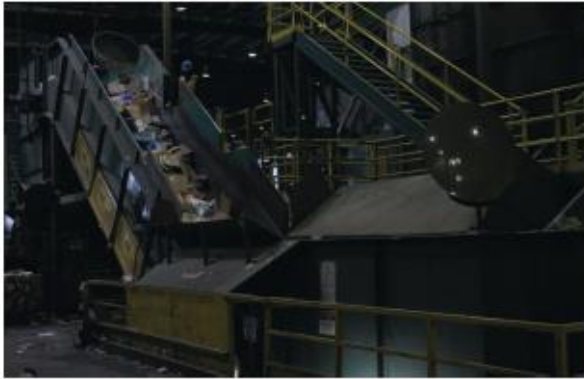
Before: Light fixtures with 400W bulbs
